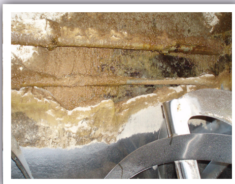
Figure 3: corrosion on mixer cover due to caking
