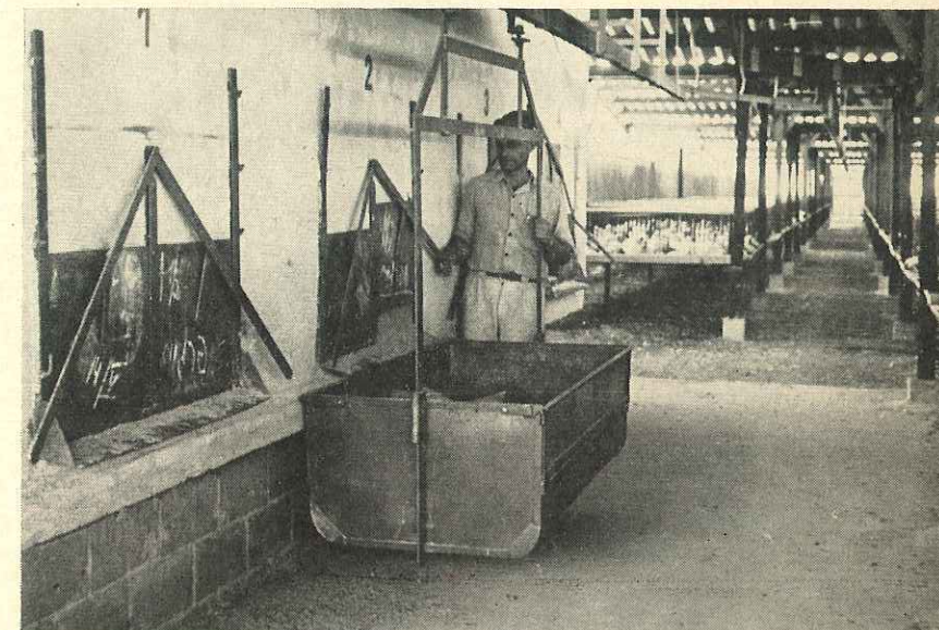
Feed carrier (above) is filled from bulk feed bin. The carrier travels on an overhead rail to ease the job of feeding the birds.
