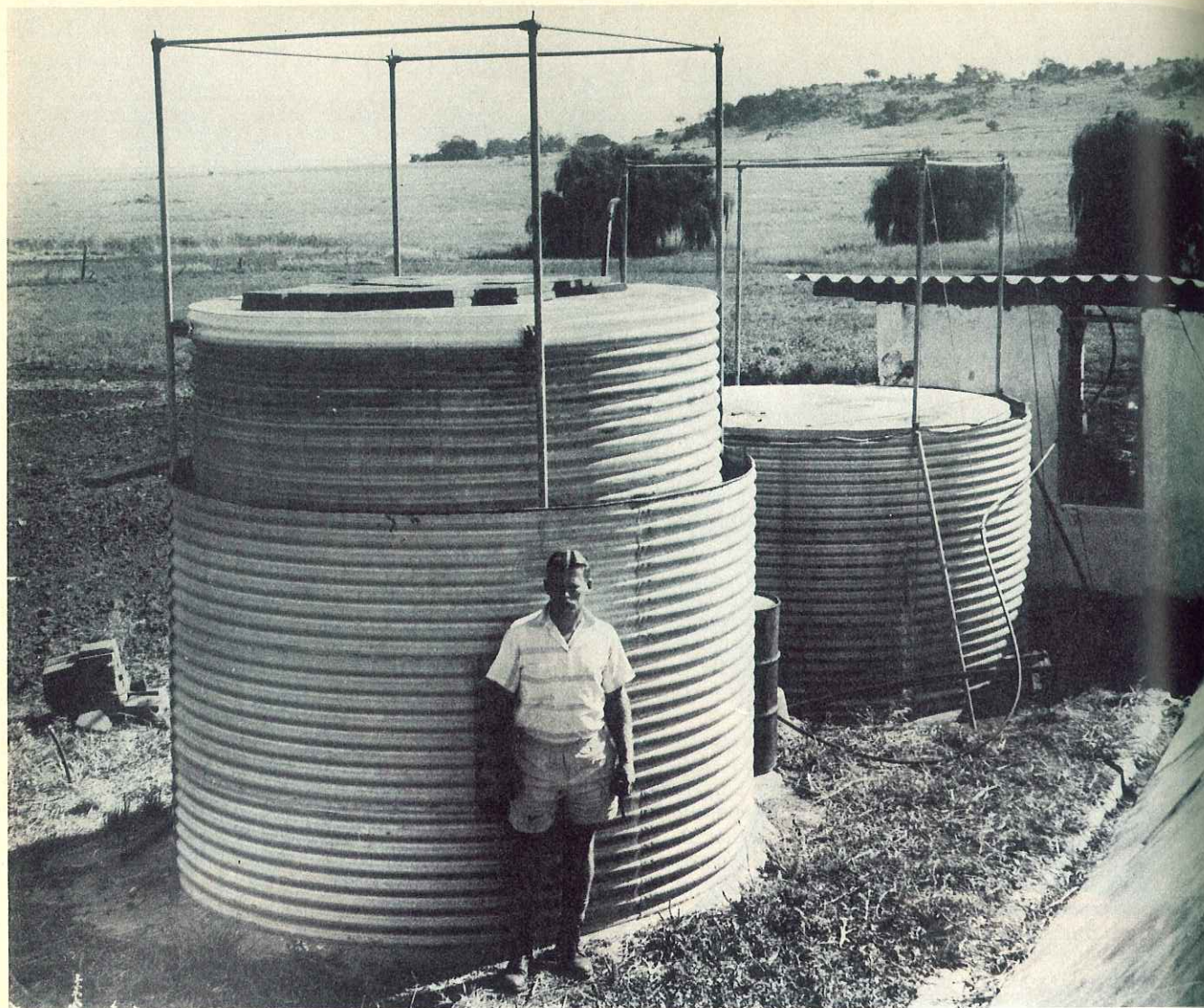
South African Mr. L. J. Fry has used this plant for over 15 years to collect inflammable gas from animal waste. The gas powers a converted diesel engine, heat from which is recycled to maintain the temperature in the manure digestion tank.
