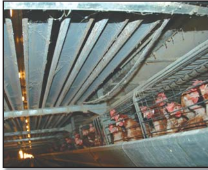
El Granjero tunnel ventilation house.
