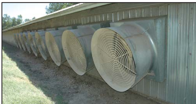
A tunnel ventilation house at the Lemus-O'Byrne farm.
