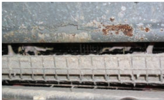
Corrosion damage from cooling pad droplets.
