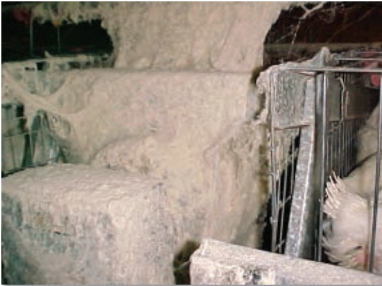
Under this mass of cobwebs is a motor that will over-heat and fail.
